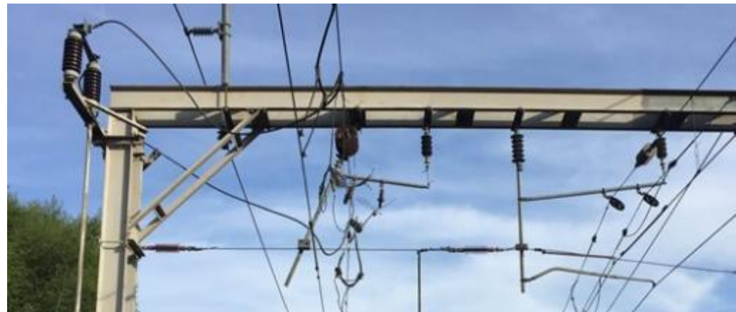
Managing our Overhead Line Equipment (OLE) is crucial to our performance.
