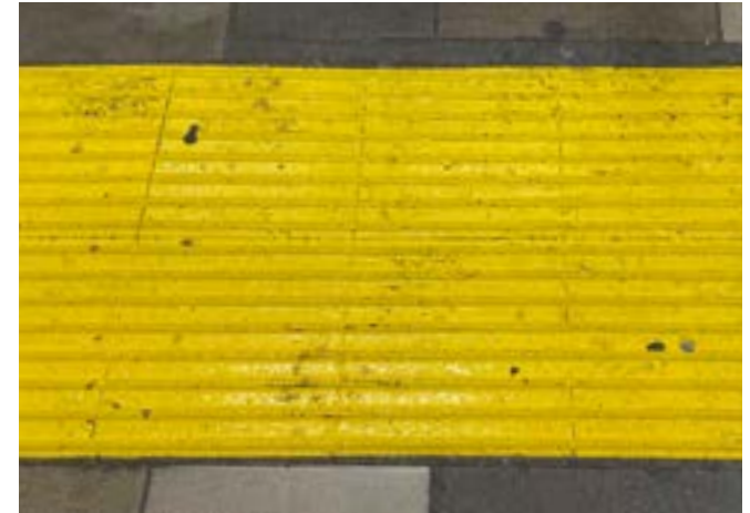
Image 4.3.3.1: Painted finishes should be avoided entirely
