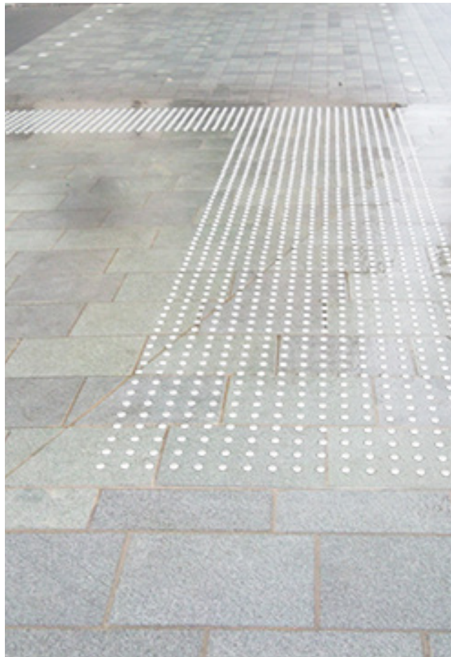
Image 4.6.1.1: Studded tactile installation in conservation area public realm in York (note that this example provides poor colour contrast).
