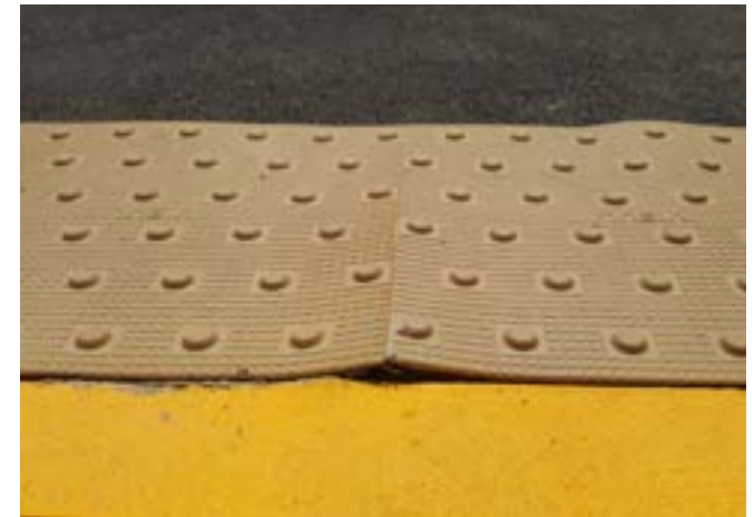
Image 4.7.6.1: Defective installation caused by lack of appropriately spaced joints
