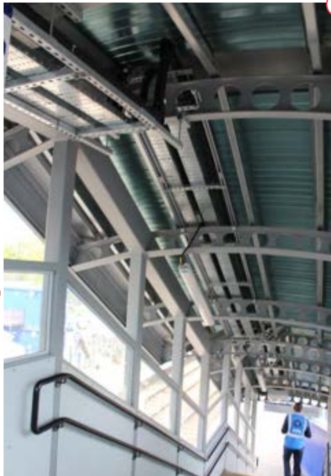
Image 7.21 Poor integration of the lighting and service runs with the structural design, and an excess of services, that could have been grouped into a combined CMS and set out better.
