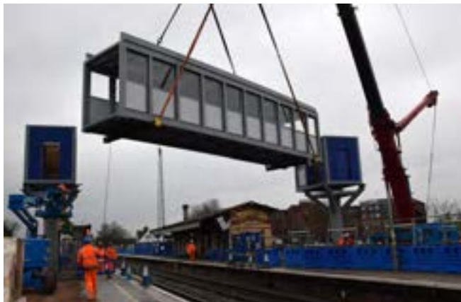
Image 6.22 Footbridge element being connected to pre-installed base elements at West Drayton station.
