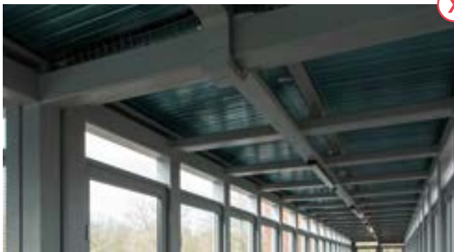
Image 7.20 CMS should not duck and dive under structure, consider castellated beams or cut outs. An integrated CMS lighting boom would have further improved this installation.
