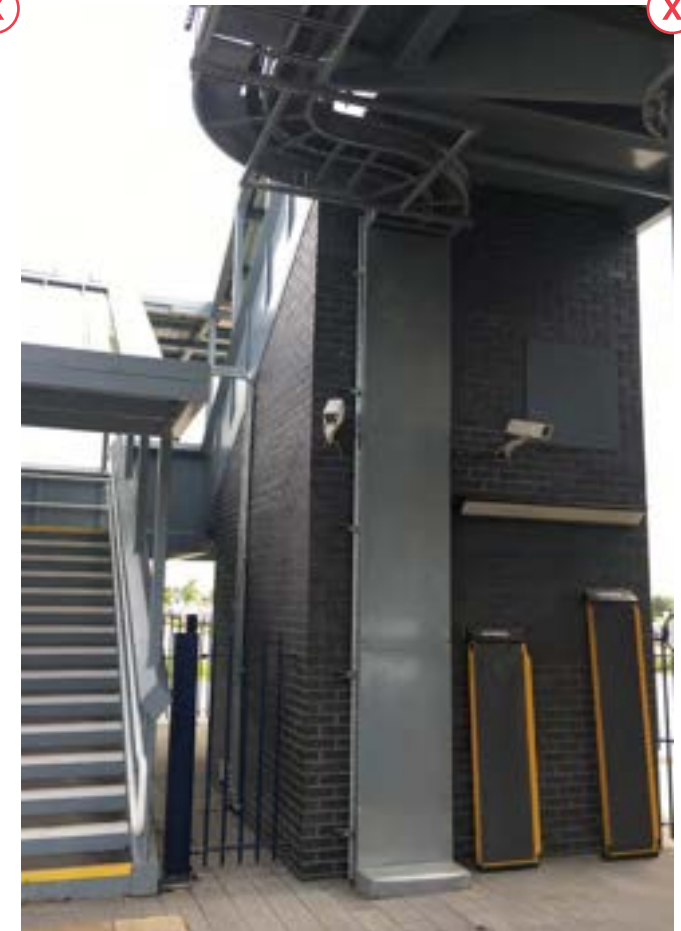
Image 7.22 Vertical service routes not integrated with the design. Services should have been considered earlier in the design. This is particularly poor as the services are located next to a plant room.
