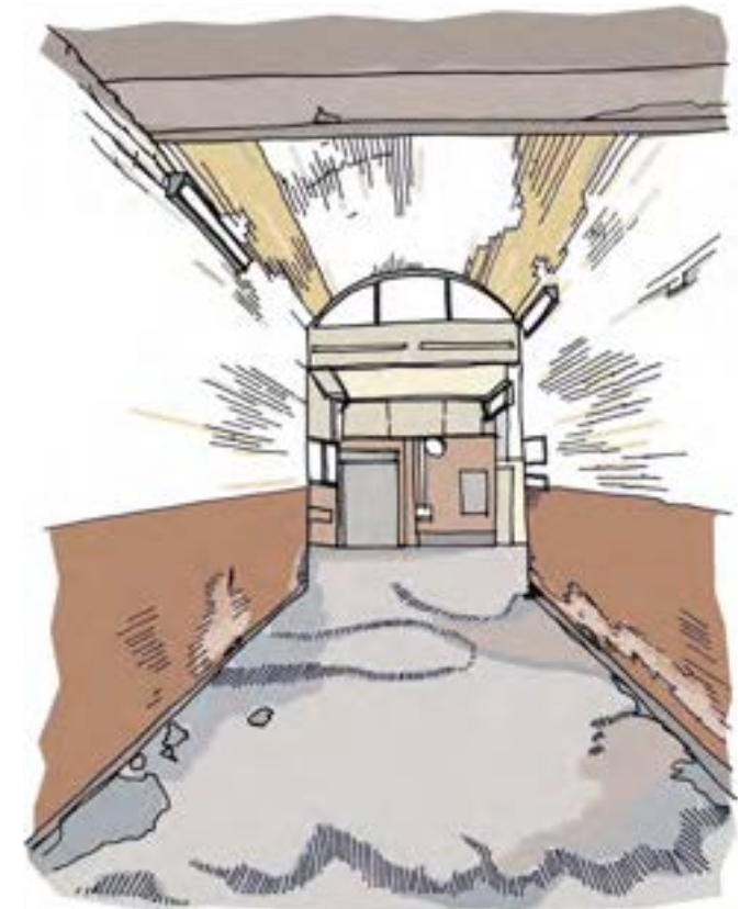
Image 8.8 Existing elements in need of care: At this station glazed bricks have discoloured due to water ingress, with stain damage at high level, and phosphorescence to the bricks below dado height.
