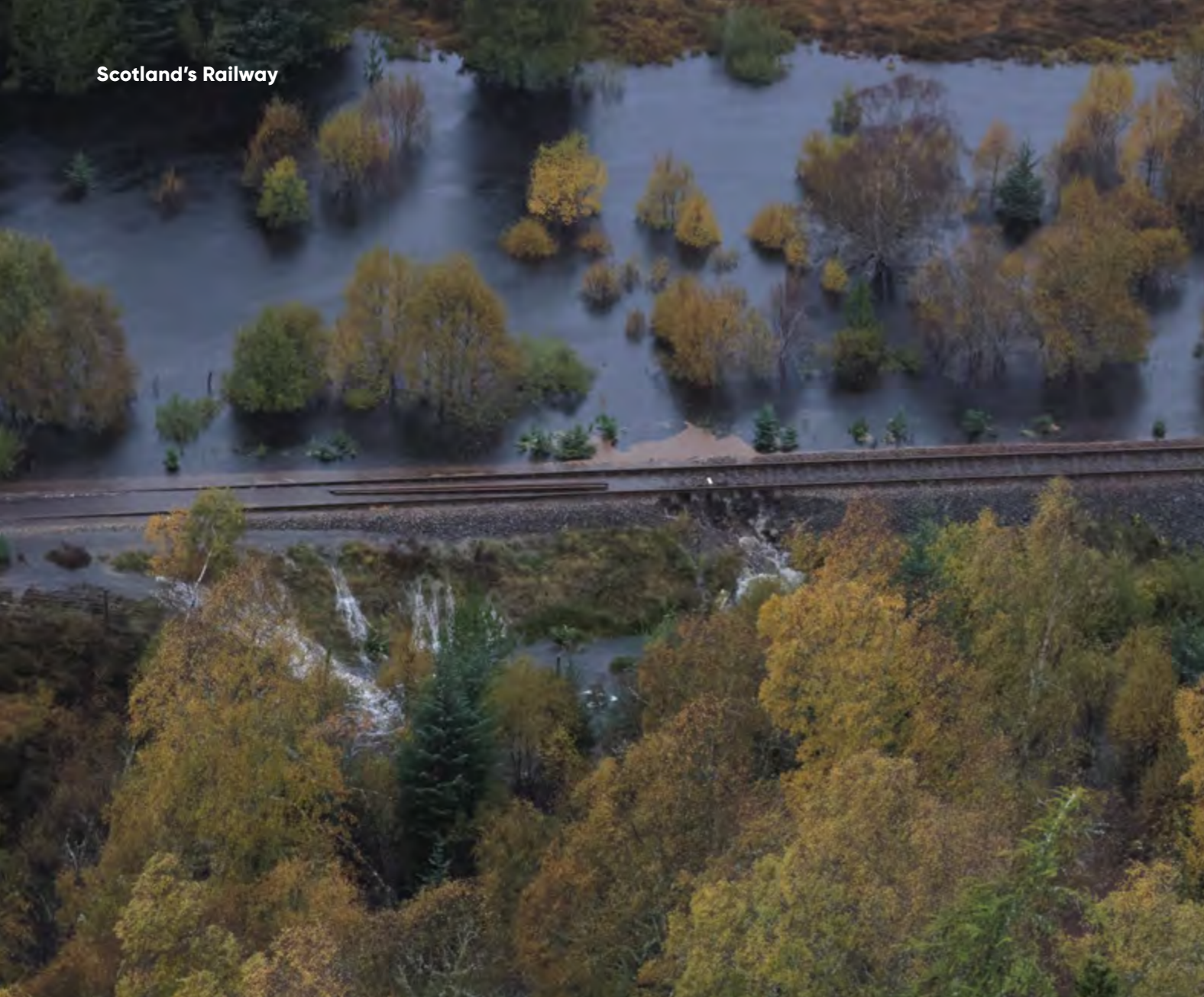
Washout event, Kyle Line, 2023
