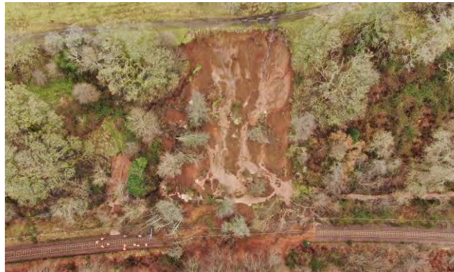
Figure 161: Fairlie landslip site
