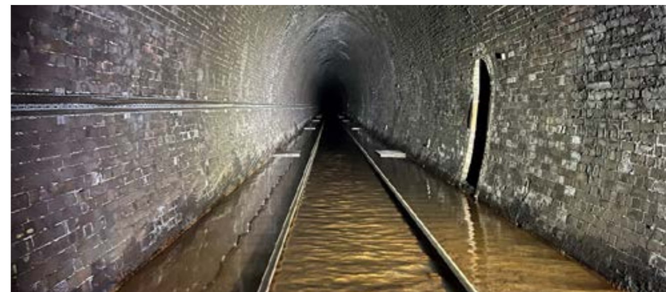
Figure 34) Water ingress at Whitehaven Tunnel Source: Whitehaven railway tunnel testing to seek source of mystery orange water (networkrailmediacentre.co.uk) Credit: Network Rail.
