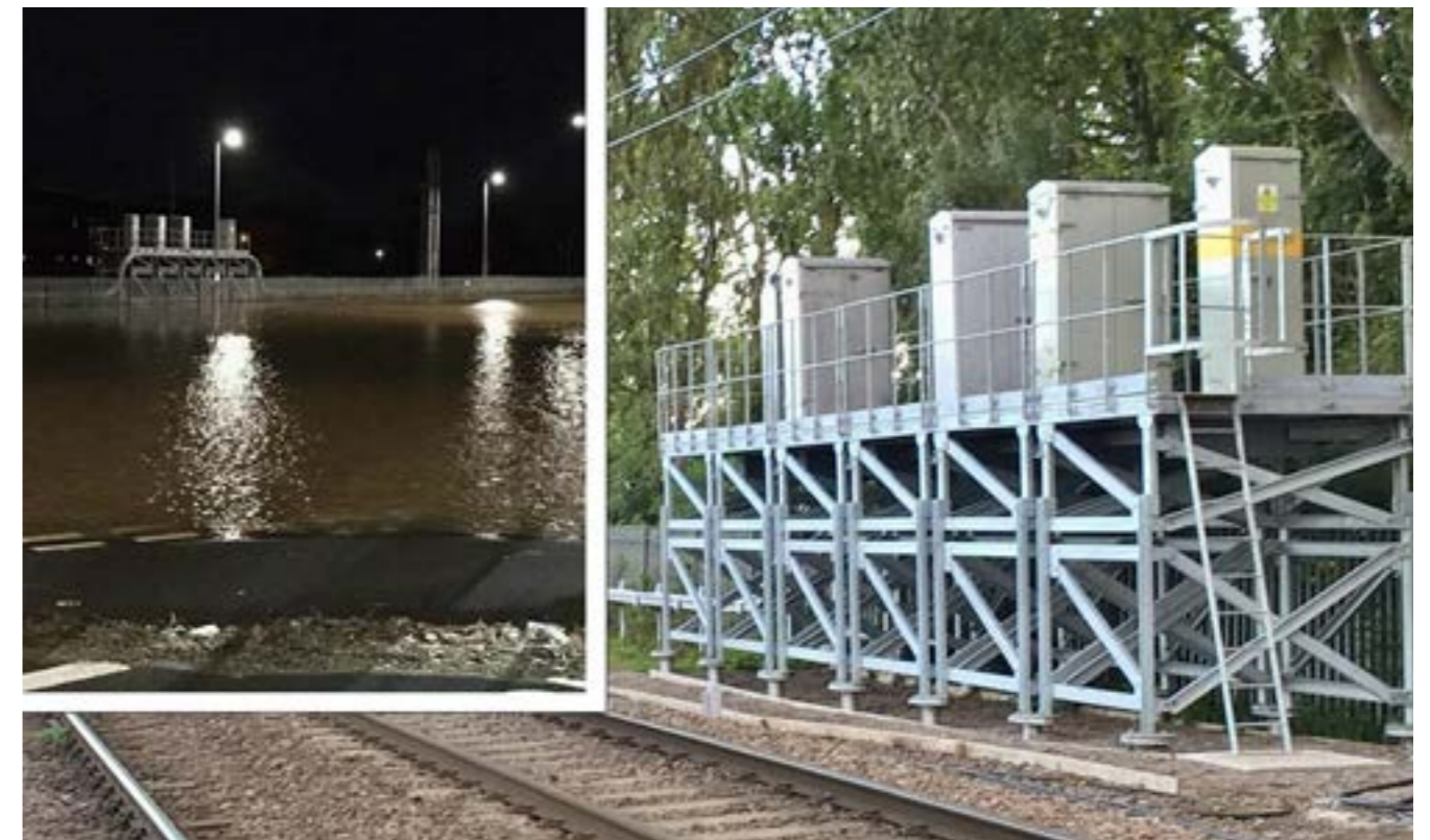
Figure 29) Signalling cabinets on stilts at Caldew junction (N. Carlisle) Source: Signalling equipment on stilts helping storm-proof West Coast main line (networkrailmediacentre.co.uk) Credit: Network Rail.
