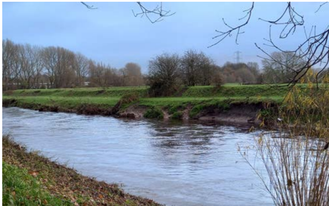
Figure 27) A river Mersey flood defence embankment offering protection to the New Mills and Cheadle Branch line (NMC) Close inspection of the flood defence mound shows signs of erosion Source and credit: Network Rail.
