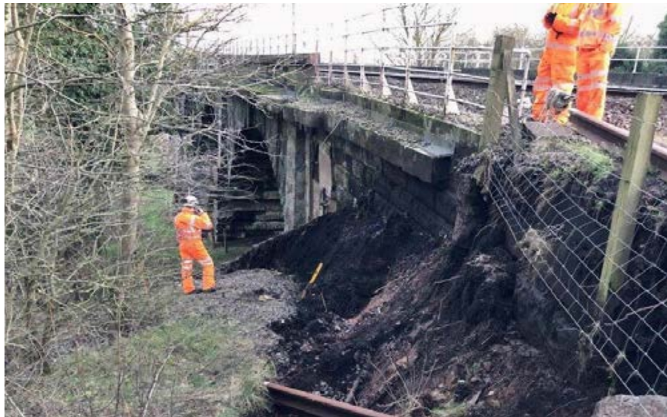
Figure 33) Landslip at Dutton Viaduct near Warrington. Source: Railway landslip forces section of West Coast main line near Warrington to close (networkrailmediacentre.co.uk) Credit: Network Rail.
