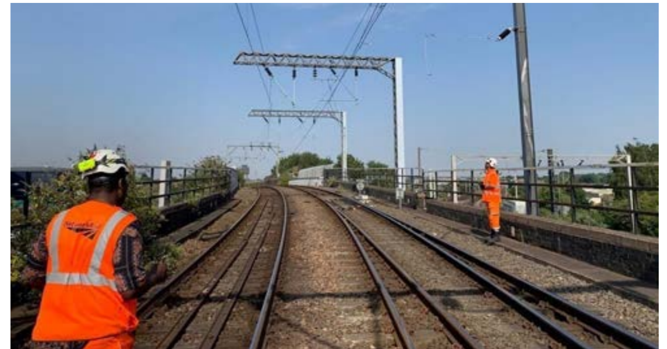
Figure 14) Site crew inspect OLE after heat damage in Birmingham. Source: Birmingham New Street trains resume after heatwave damage (networkrailmediacentre.co.uk). Credit: Network Rail
