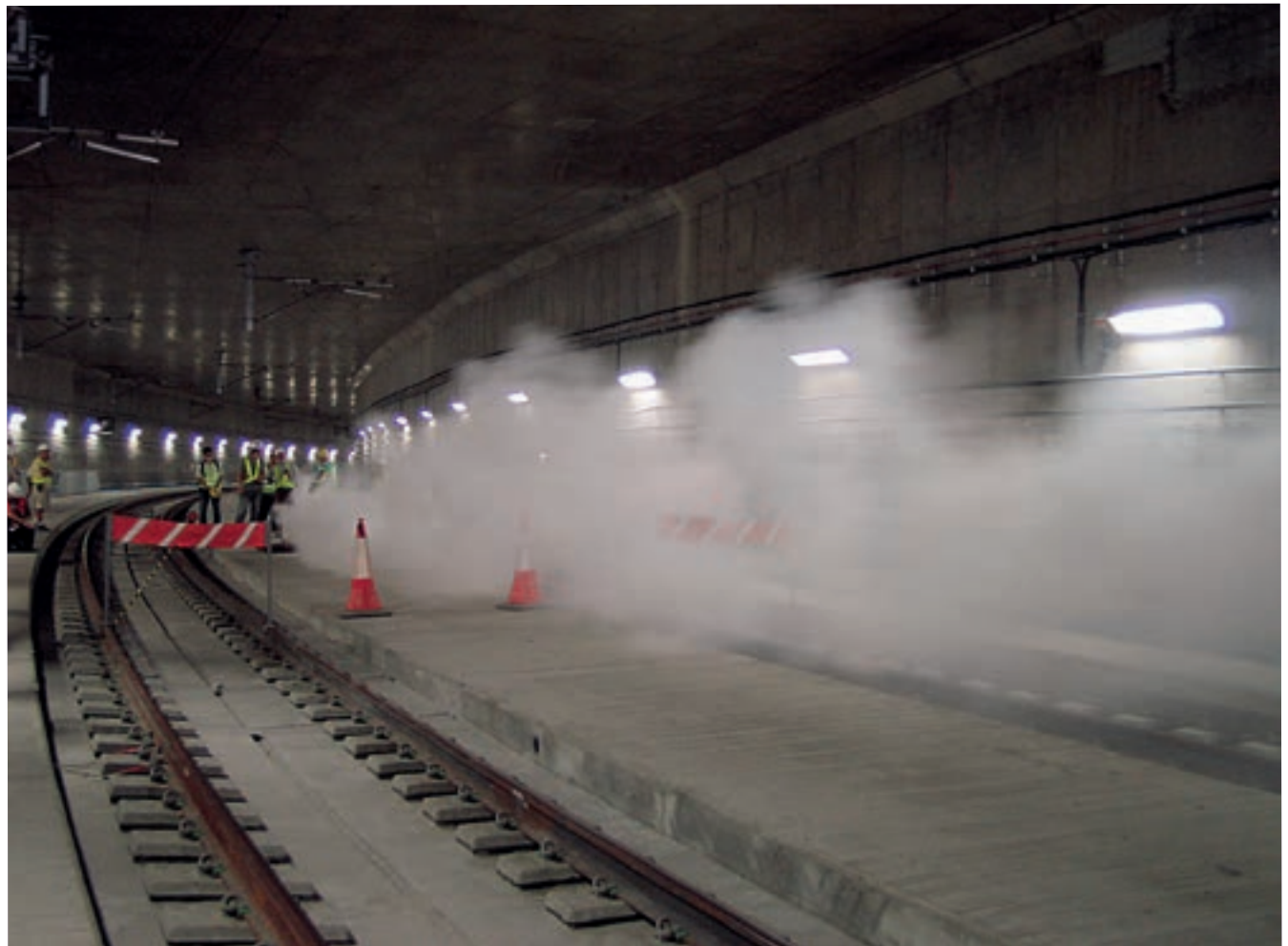
Image 7.7 Smoke ventilation testing as part of the KCRC East Rail Extension, Tsim Sha Tsui, Hong Kong © Arup
