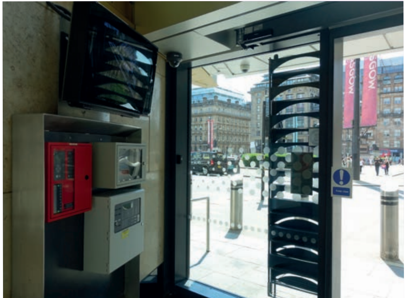
Image 8.1 Fire alarm panels at the entrance of a Network Rail station © Arup
