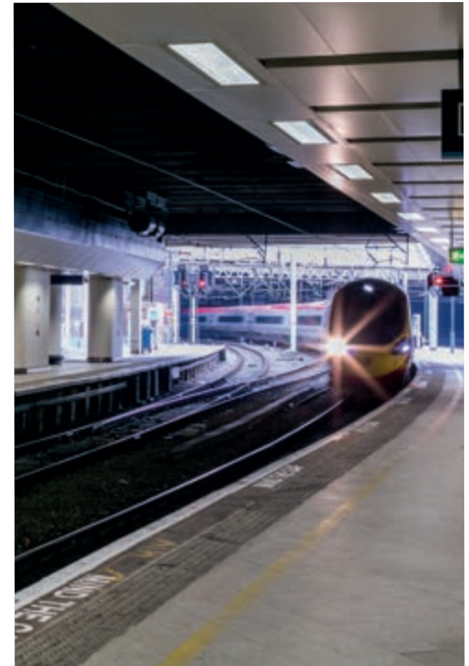
Image 8.6 Impulse smoke fans serving sub-surface rail lines at Birmingham New Street Station © Network Rail
