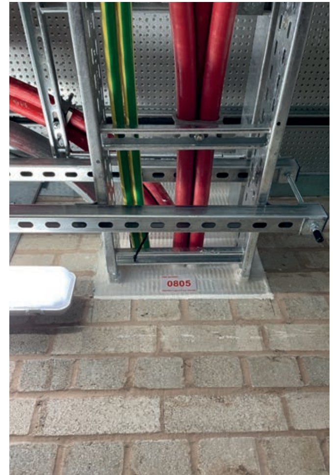
Image 5.7 Example of a cable penetration sealed with firestopping © Arup
