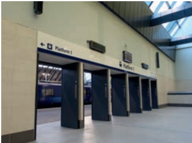
Image 5.6 Set of FD60 fire doors between Glasgow Queen Street Station High & Low Level Stations © Arup
