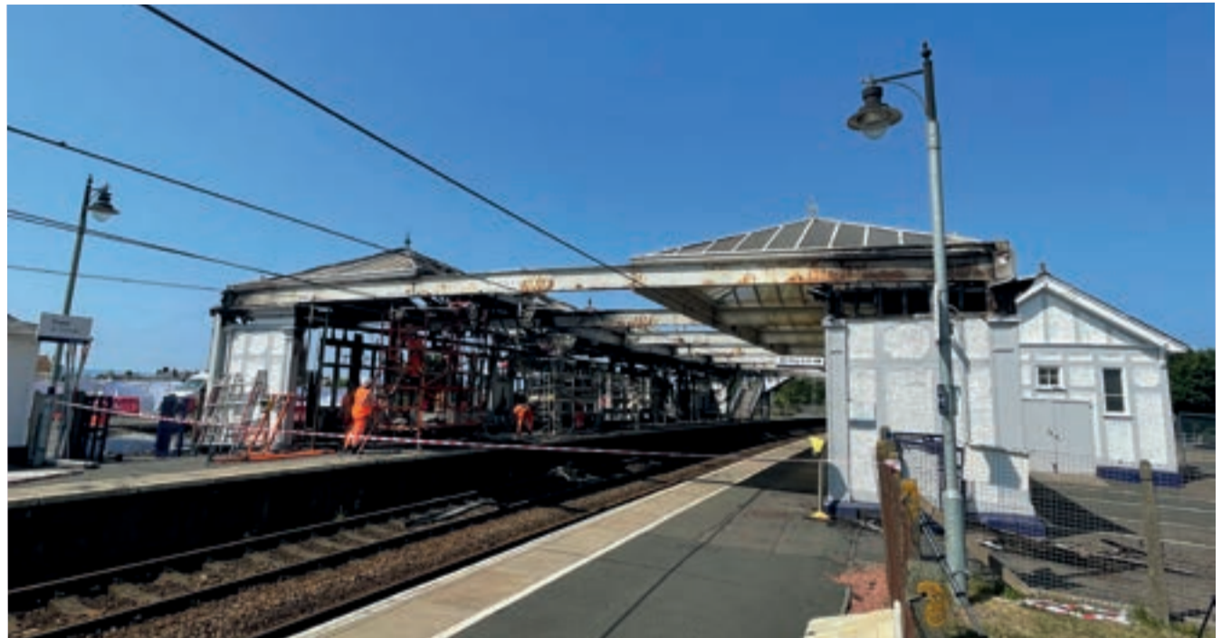
Image 8.2 Aftermath of the fire at Troon Station © Network Rail
