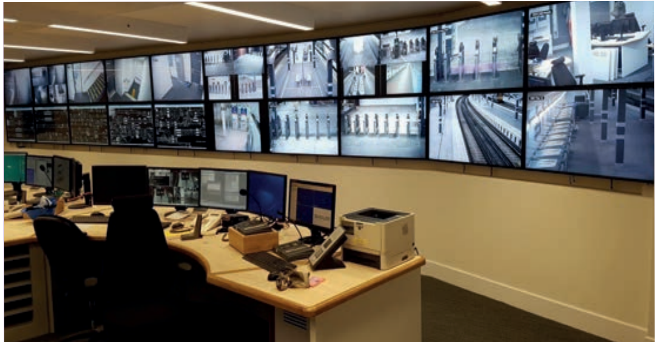
Image 7.5 London Bridge station control room © Network Rail
