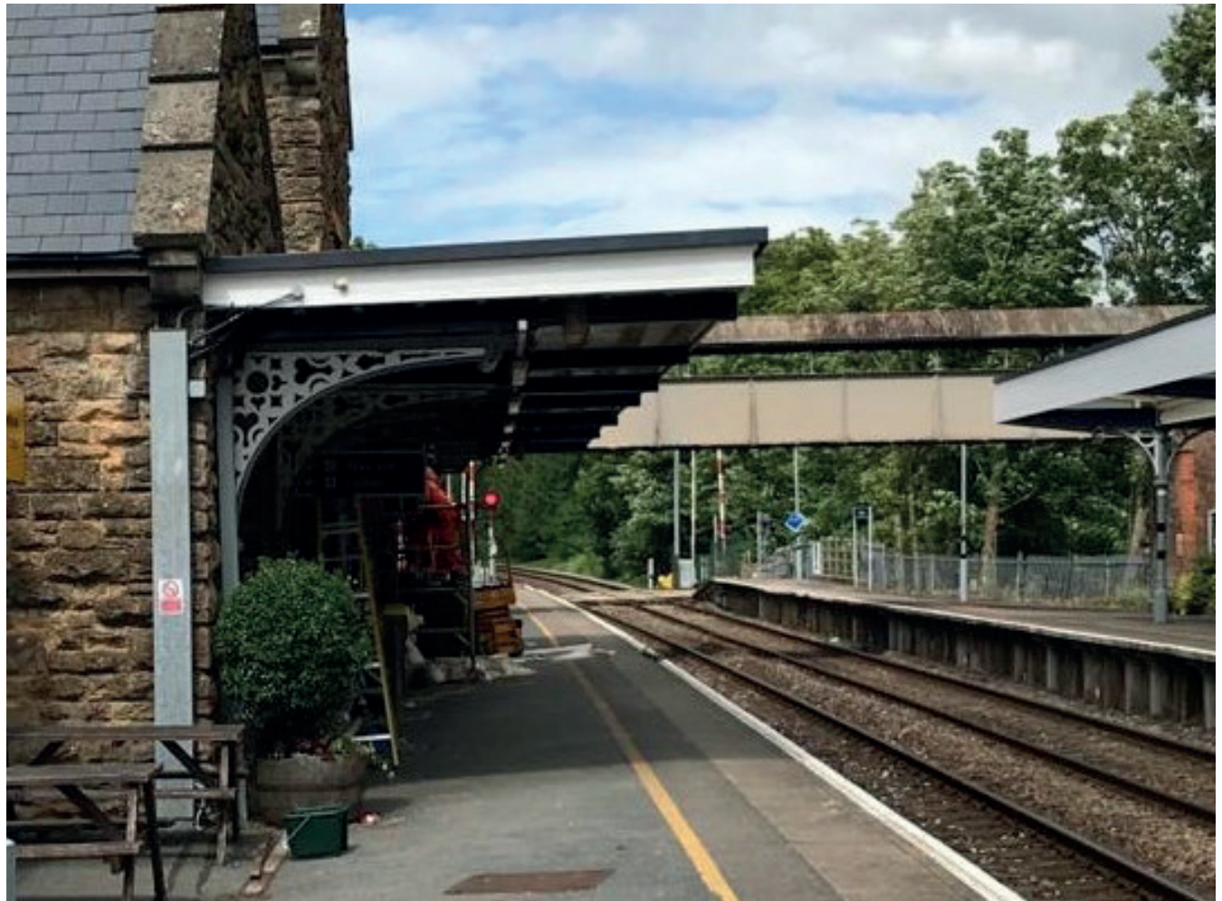
Image 4.3 Existing stations like Sherbourne Station may have limited improvement options © Network Rail
