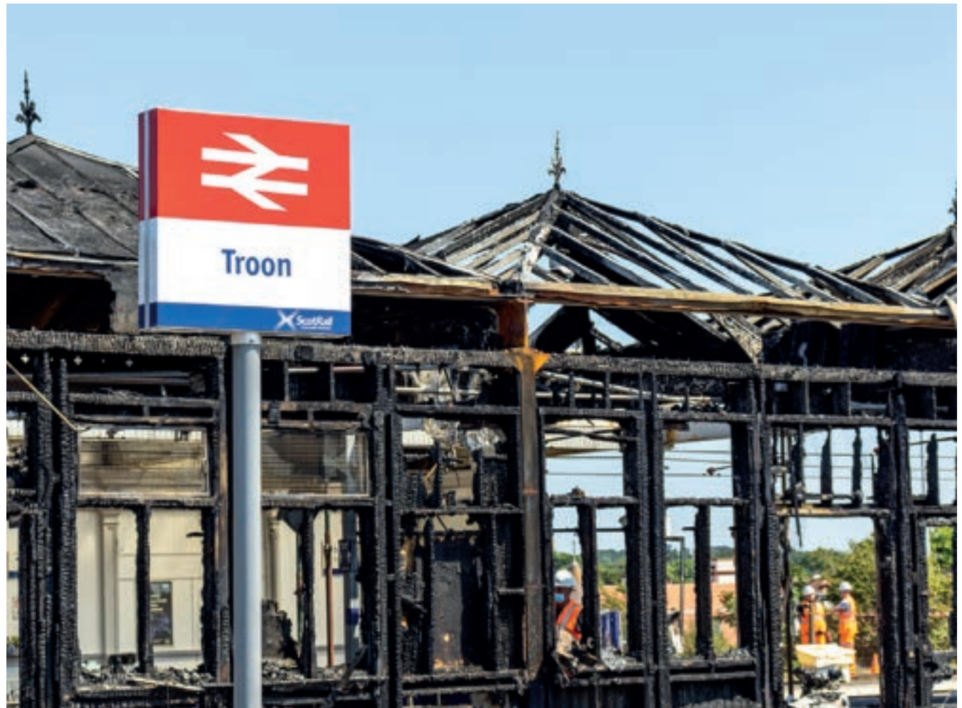
Image 2.2 Troon Station Fire © Network Rail
