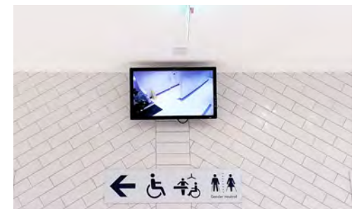
CCTV monitor in WC entrance at London Victoria. Image: Oliver Ansell
