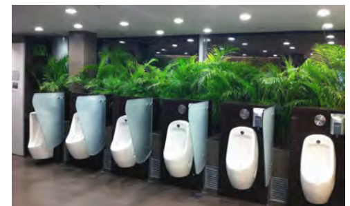
Planting within Singapore Changi Airport. Image: Mark Miller. Note that all planting to be behind glass in stations.
