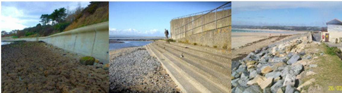
Figure 3-2: Examples of vertical wall (left) and stepped concrete and rock revetments (centre and right)
