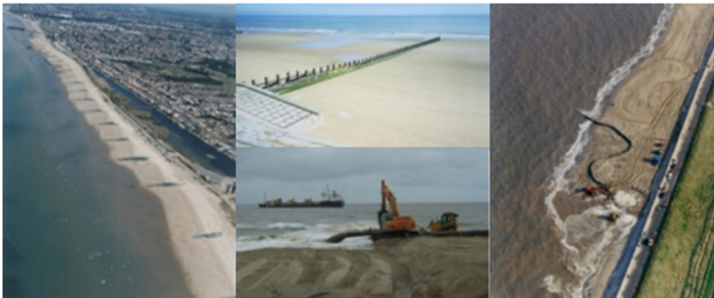
Figure 3-5: Images of beach management and control structures
