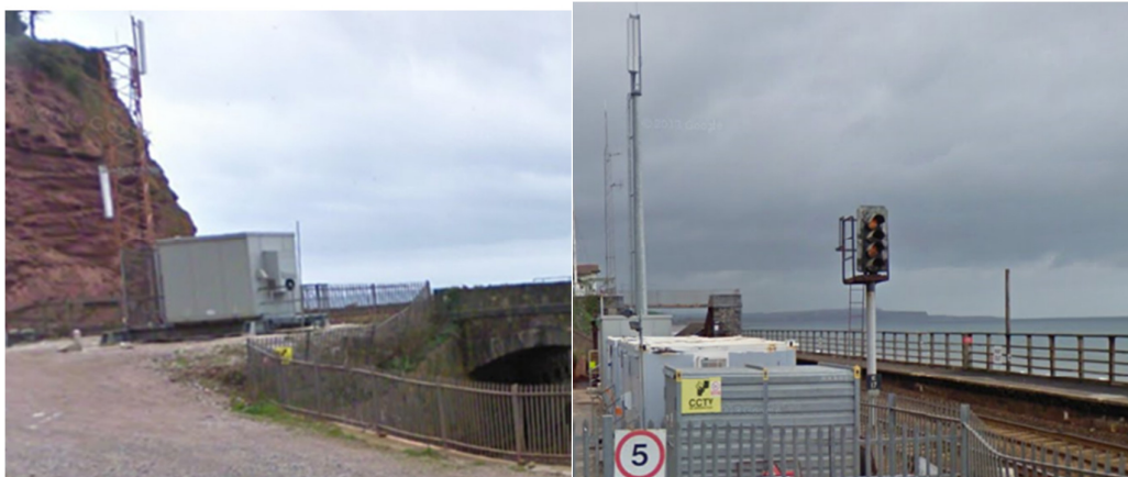
Figure 3-23: Equipment building and mast at Smugglers Lane (left panel) and mast within Dawlish Station compound (right panel)
