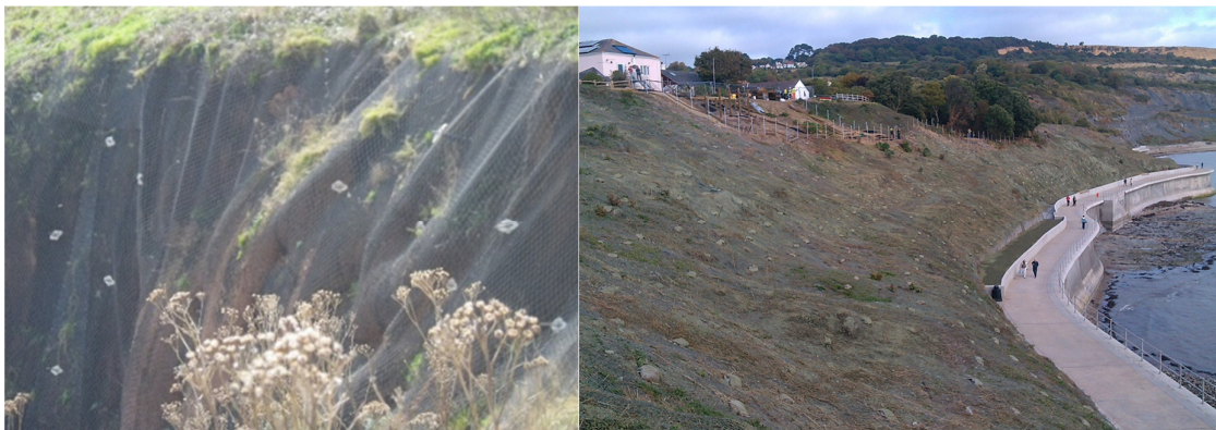
Figure3-8: Left – Soil nailing and meshing at Windjammer (CBU11) and at East Cliff, Lyme Regis
