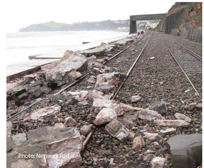
Damage following the February 2014 storms at Dawlish
