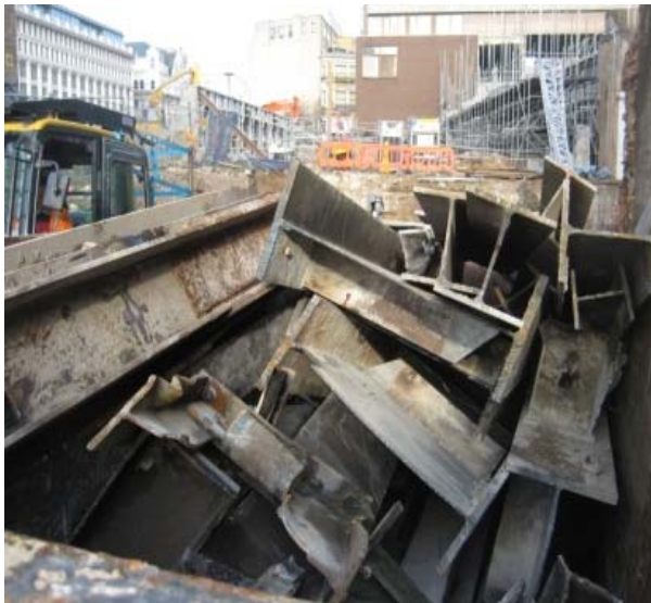
Steel is segregated on-site where possible. When noise constraints occur the separation can take place off site.
