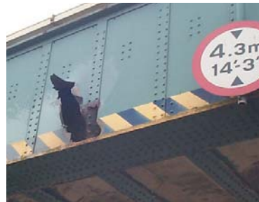
Damage caused to a bridge by an unsecured equipment arm
