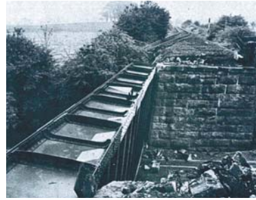
A bridge strike can seriously damage railway bridges
