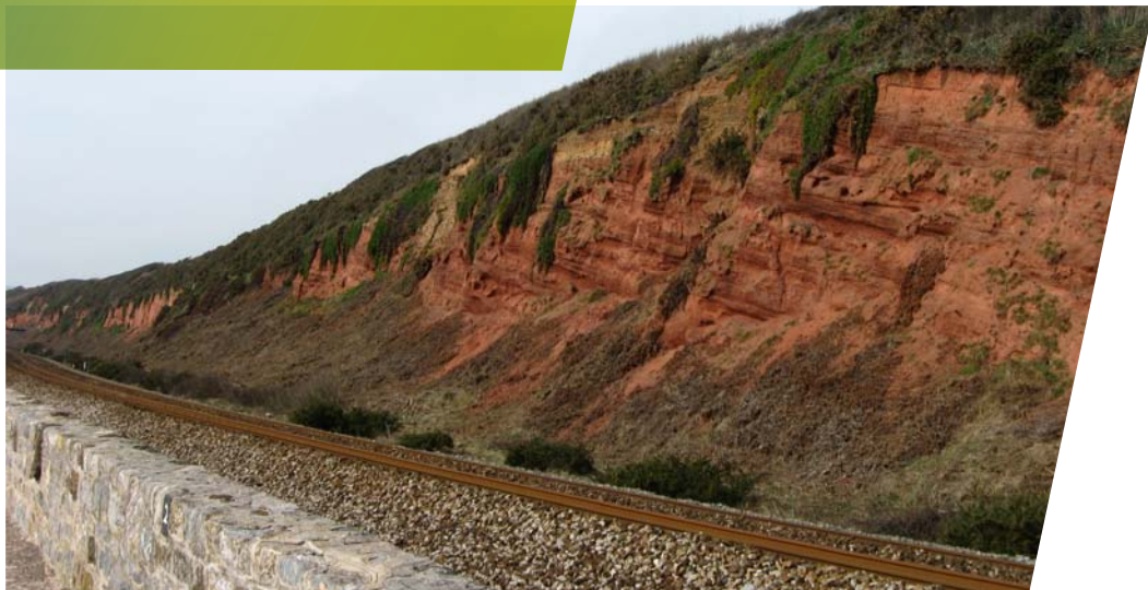
Dawlish Cliffs after works have taken place showing where the Hottentot fig has died.
